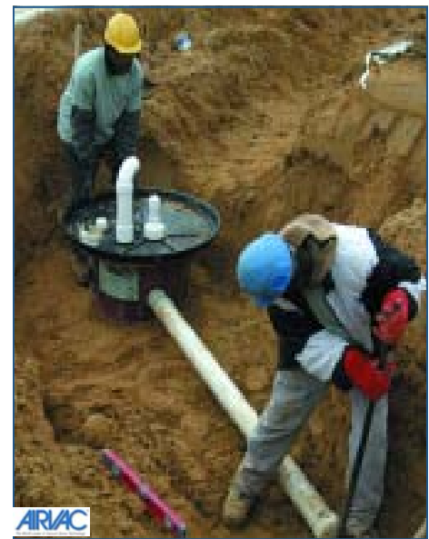
A valve pit is installed at each wastewater source.
